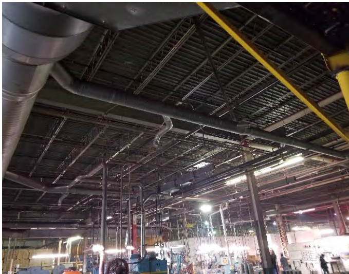
Current Weld Line
